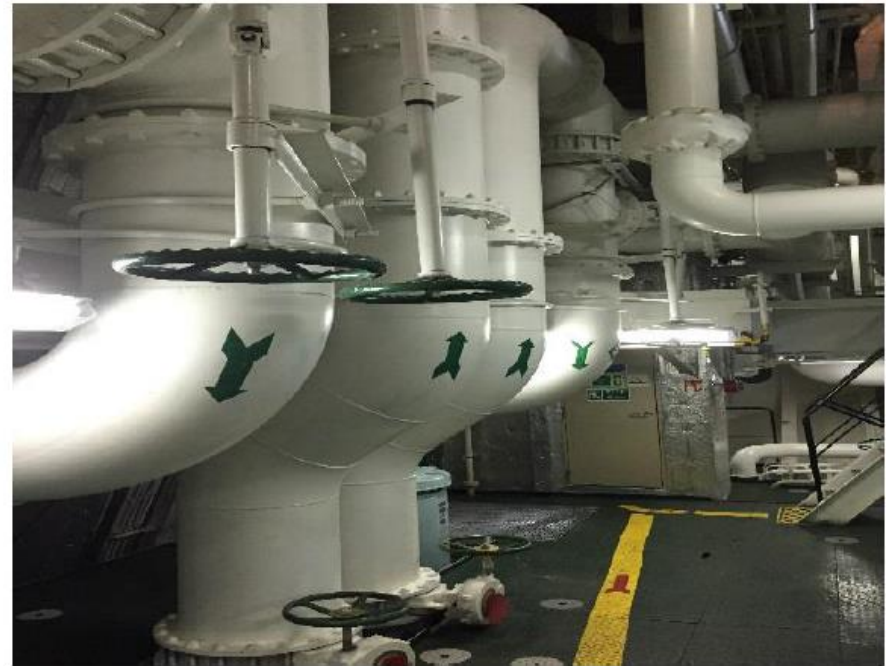
BWTS Piping in Engine Room
