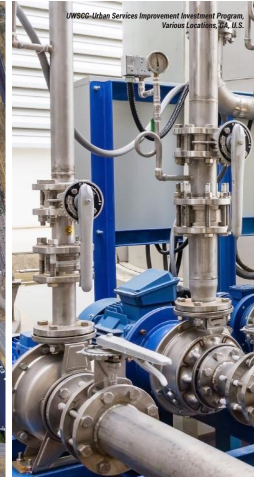
Sacramento Regional Wastewater Treatment Plant EchoWater Project, Elk Grove, CA, U.S.
