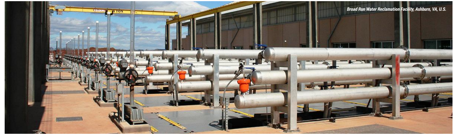
West Lafayette Water Treatment Facilities, West Lafayette, IN, U.S.
